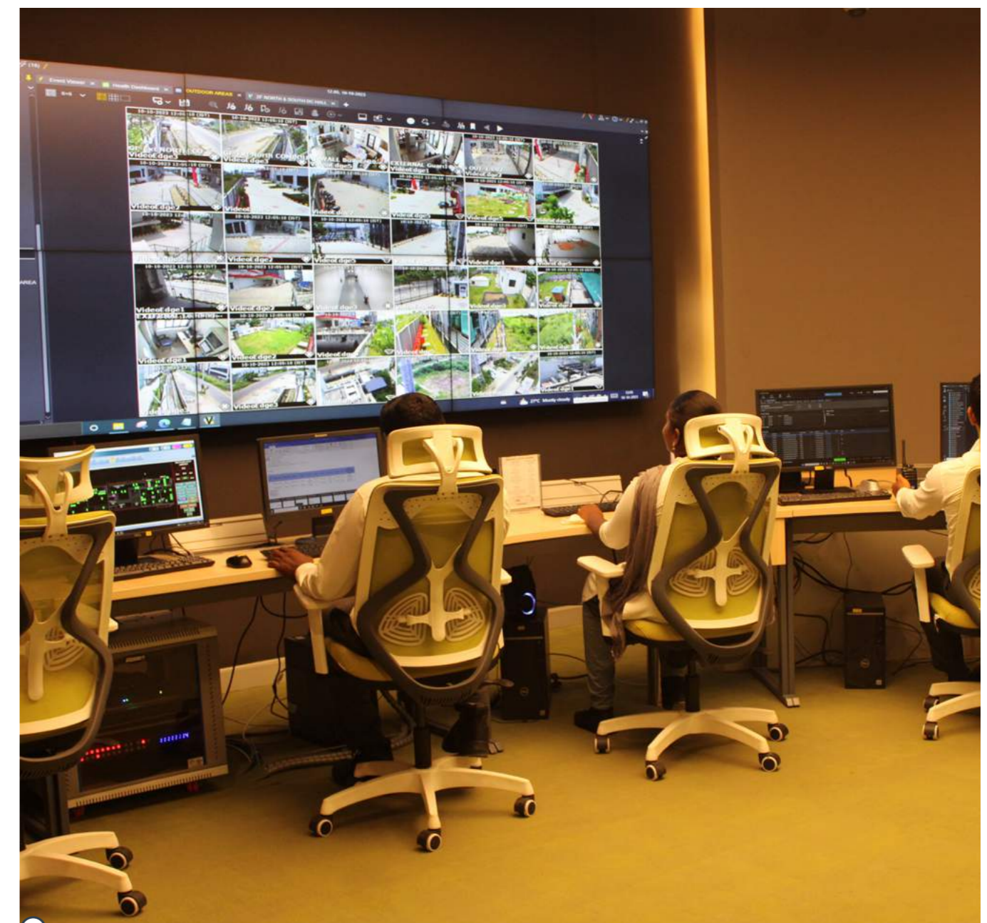
Security Operations Centre at one of our data centres in Chennai
